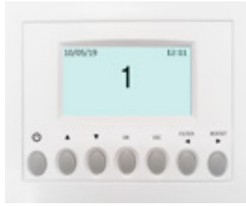
Fig. 7.d CTRL-DSP operation screen
